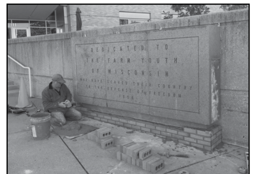
The plaque honoring Wisconsin farmers serving in the military was re-installed at DATCP.
